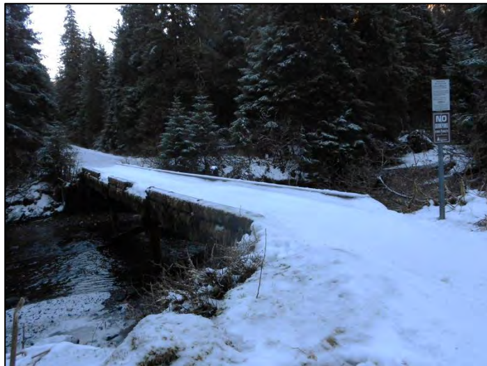
Figure 30. The Montana Creek Bridge located at the end of Montana Creek Road. Photo courtesy of Amy Sumner, JWP.
