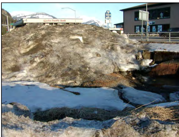
Figure 42. Snow being stored near Jordan Creek at Glacier Highway. The snow has been pushed into the creek and is depositing sediment in the streambed. Photo from JWP's archives.
