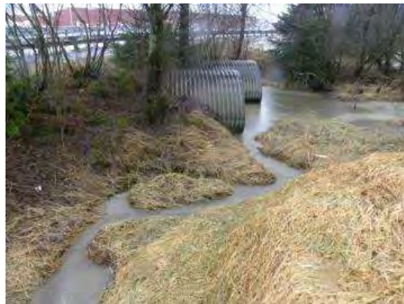
Figure 22. Turbid stormwater discharges to Jordan Creek from the Crest Street ditch near Yandukin Drive. Photo Courtesy of John Hudson.
