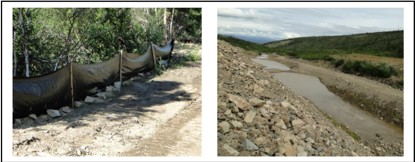
Examples of best management practices. Silt fence (left), elongated sediment ponds (right)
