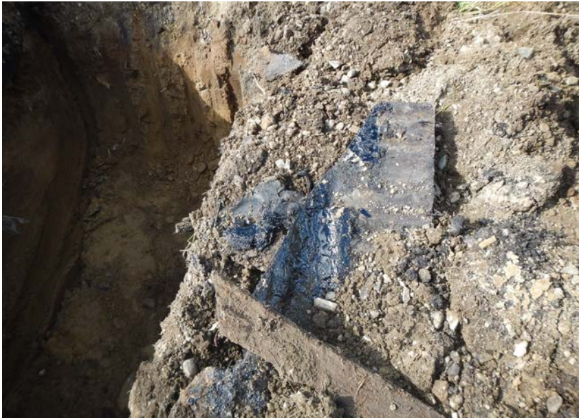
Photo 10: Fuel-coated wooden debris was encountered adjacent to the Test Pit 1 and in Test Pit 4 on the Property. (August 29, 2014)
