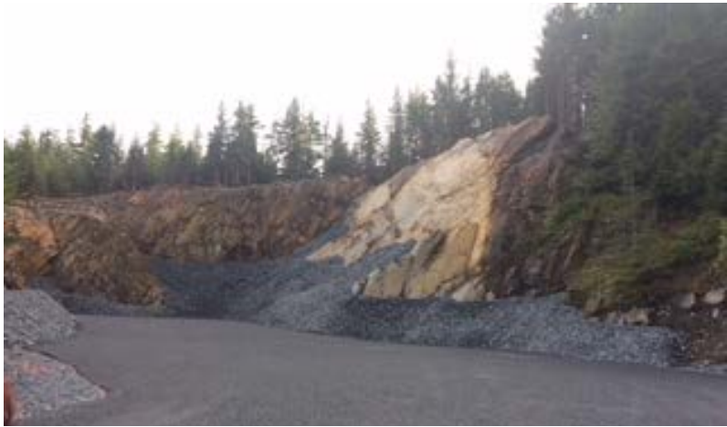
Figure 6. Rock Pit #2, prepared for soil placement. Aggregate has been placed on the floor of the quarry to create a smooth surface for soil placement. Some Chimney Rock for drainage has been placed. Photo by Chris Hatton, Wrangell Cooperative Association IGAP.
