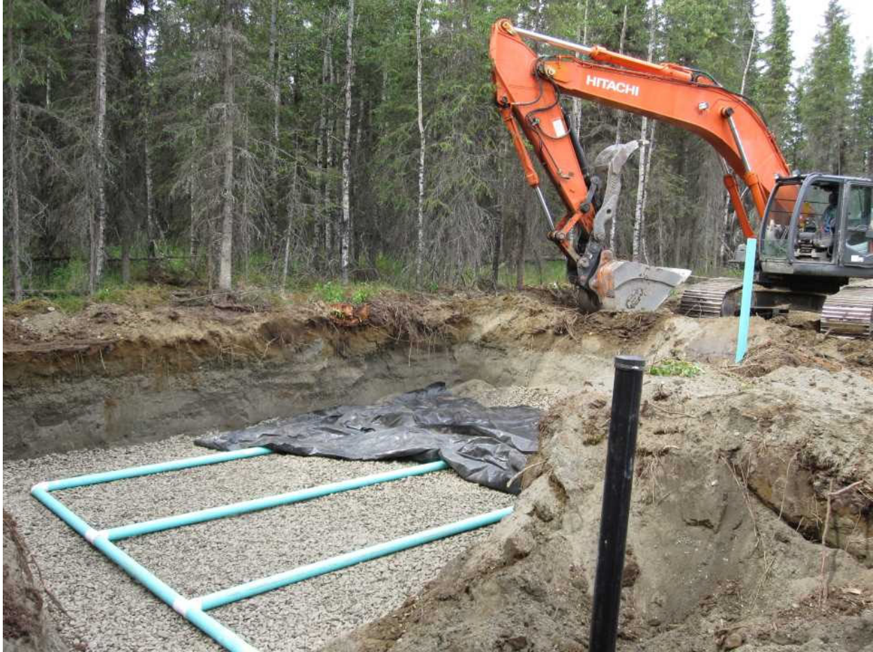
Conventional bed type leach field being installed. Photo taken by DEC staff.
