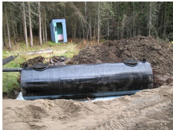
New onsite wastewater system replaces pit privy. Photo taken by DEC staff.
