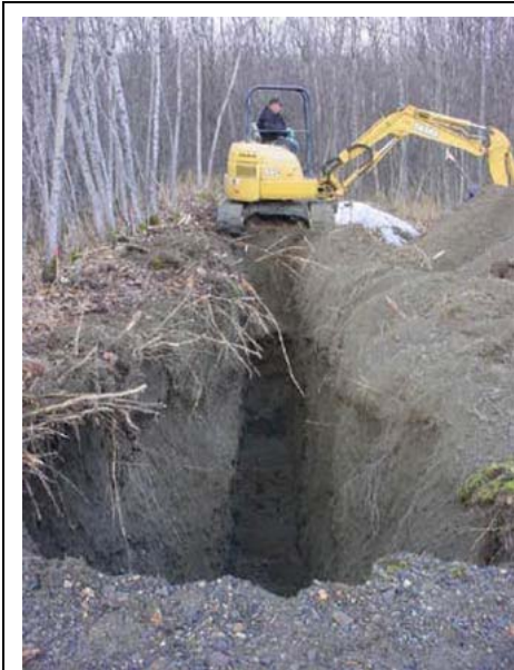
A septic trench dug in Aniak October 2006 allow sampling. Results showed soil and groundwater contamination. We also learned that vapors from the contamination are entering the air inside buildings at levels which are low but exceed state and federal target levels.
