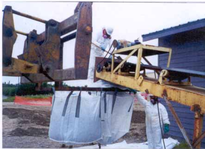
Photo 2: A forklift was used to support the supersacks while they were being filled with PCB impacted soil.
