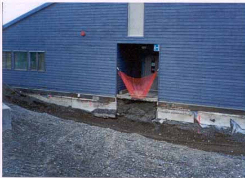
Photo 4: This is a photo of the same area shown in Photo 3 after removing several feet of PCB impacted soil. The doorway shown above is the south entrance to the Aniak Middle School.
