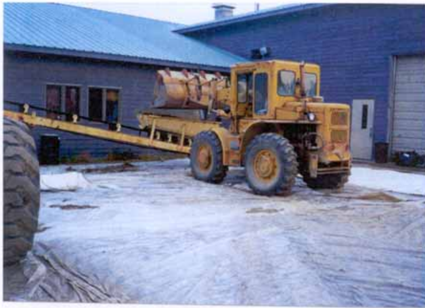
Photo 1: The front end loader is shown placing soil onto the conveyor belt. The work area was covered with a plastic liner. After the supersacks were loaded, the soil collected on the plastic liner was placed in supersacks for disposal.
