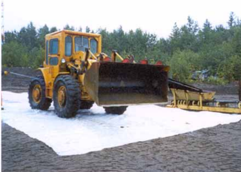
Photo 4: At the conclusion of the excavation activities, a decontamination station was set up using a plastic liner. Gravel berms were constructed on the downslope edges of the plastic liner shown above, and the rinsate from washing the equipment was collected and transferred to a 55-gallon drum.
