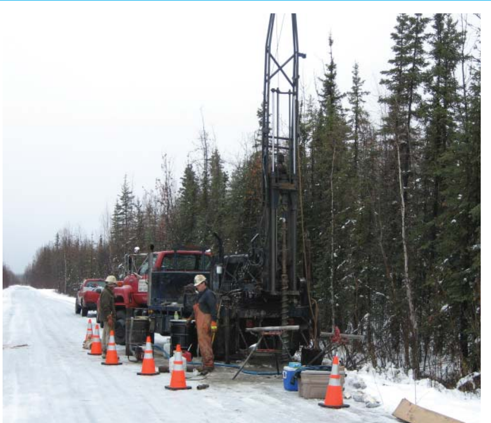
Homestead Drilling workers, shown in November, set up a drilling rig to install Monitoring Well No. 188, which is outside the plume and the farthest northwest of the refinery. It's just over 2½ miles northwest of MW No. 166, at Bradway Road and Luckies Lane. To date, it's been nondetect for sulfolane. Photo courtesy of Shannon & Wilson.
