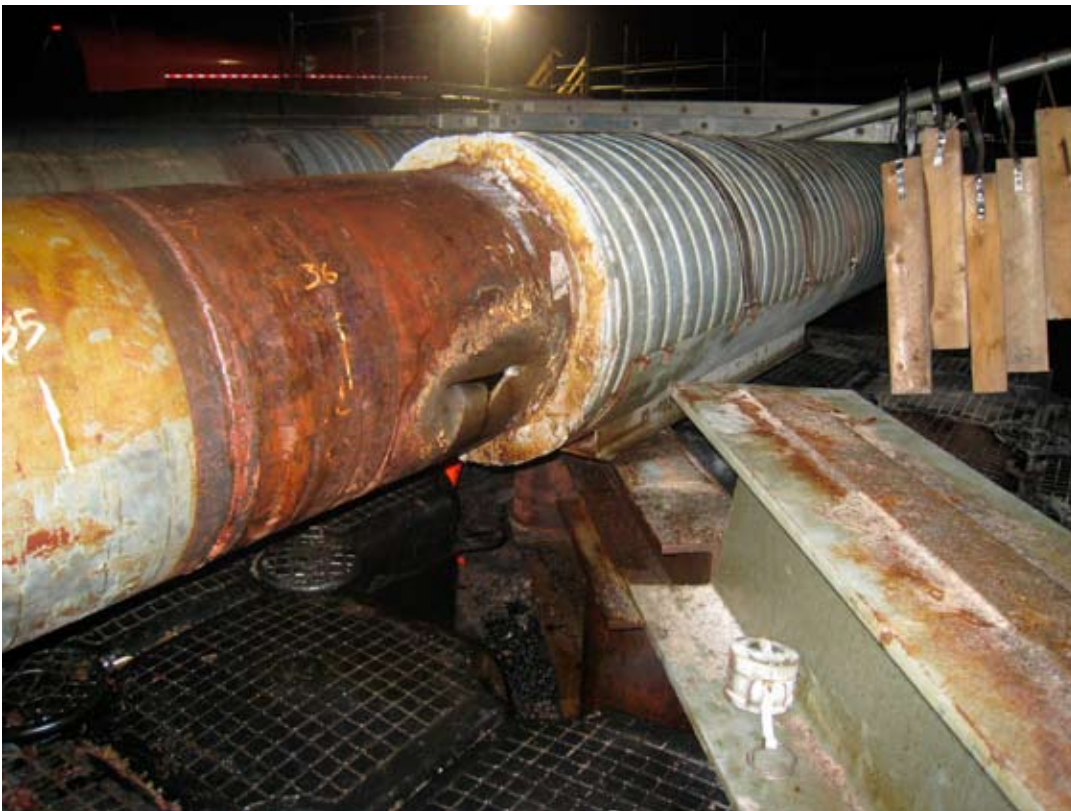
Photo showing the puncture in the BPXA DS 16 Flowline D and the wooden blocks to prevent the flowline from shifting. (Photo courtesy of BP)
