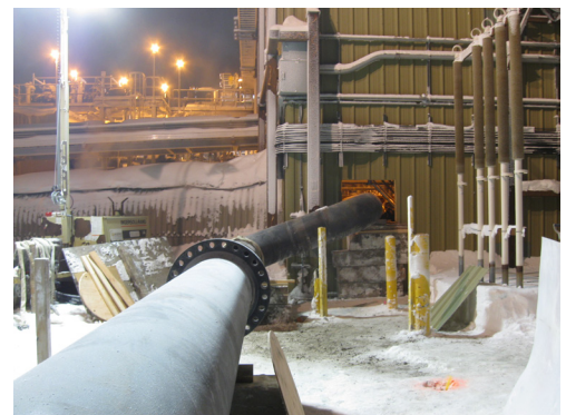
The 24-inch bypass line, under construction, enters the metering building at PS 1. (Photo courtesy of ADEC)
