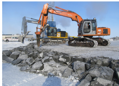
Cleanup operations at site of Repsol Q2 Gas and Mud Release. (Photo courtesy of ADEC)
