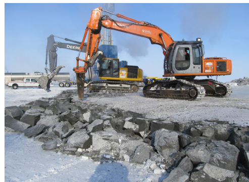
Cleanup operations at site of Repsol Q2 Gas and Mud Release. (Photo courtesy of ADEC)
