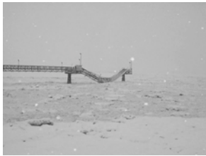
View of damaged dock
