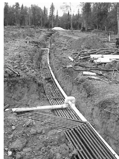
Gold Creek -- Soil Vapor Extraction system and lines being installed on the west side of the spill site.
