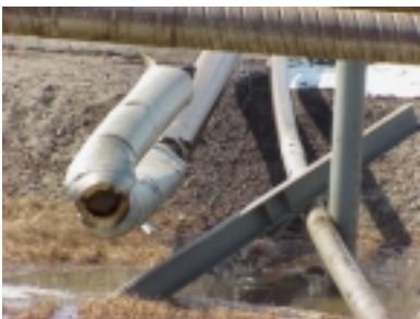
Crimped and severed pipe at ARCO Drill Site 14.
