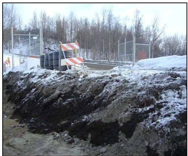
Fuel seeping into recently excavated ditchline near gated entrance to powerplant.
