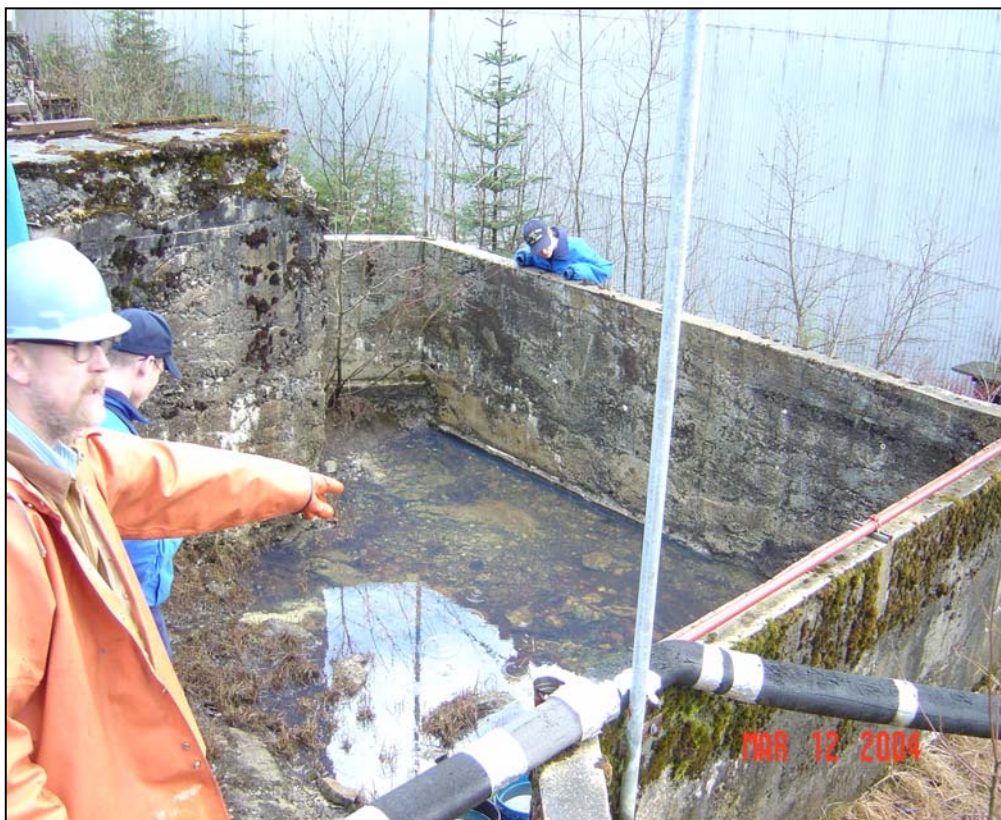
Photo 2. Diesel pooled in the containment area. ADEC Photo.
