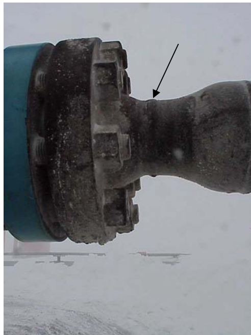
Location of failed weld on the flowline.
