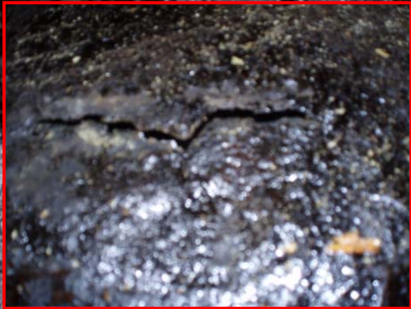
Close up of crack
