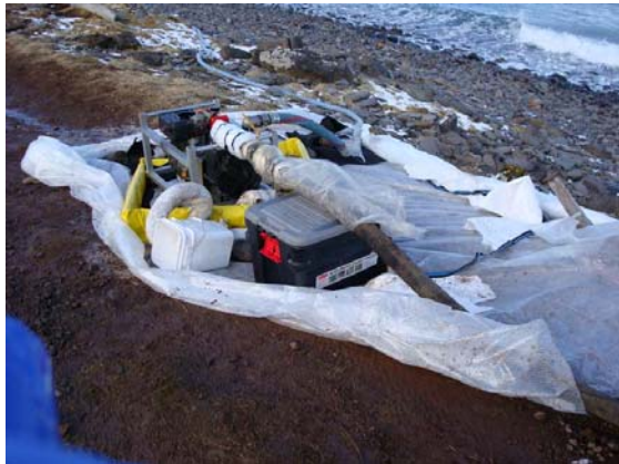
Containment around peristaltic pump on shore.
