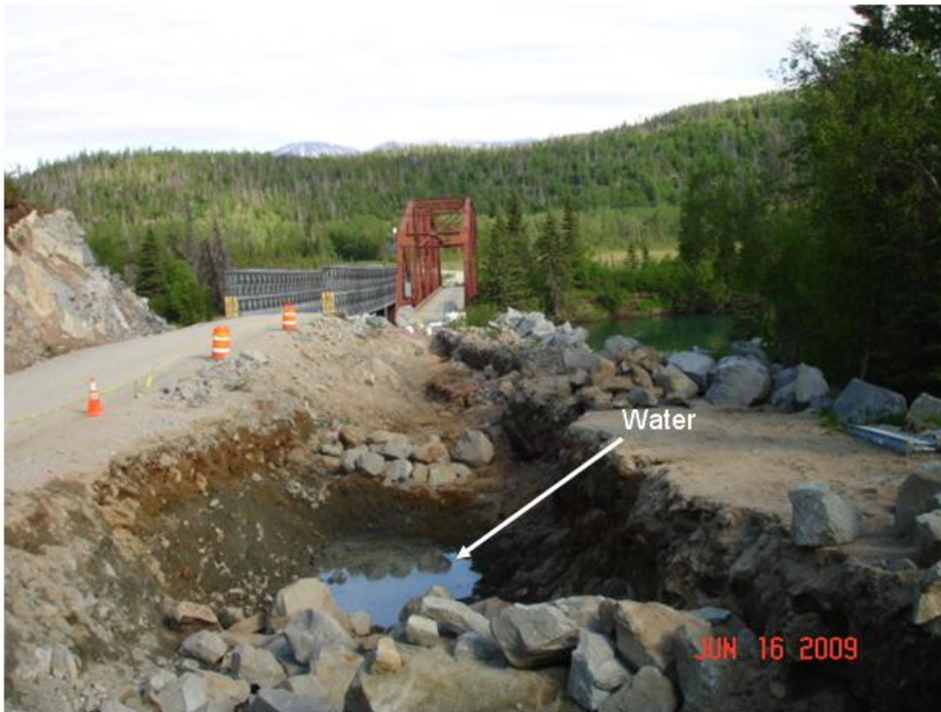
Photo of excavation area. Groundwater in the lower section of the photo shows very light sheen. Photo taken by ADEC.
