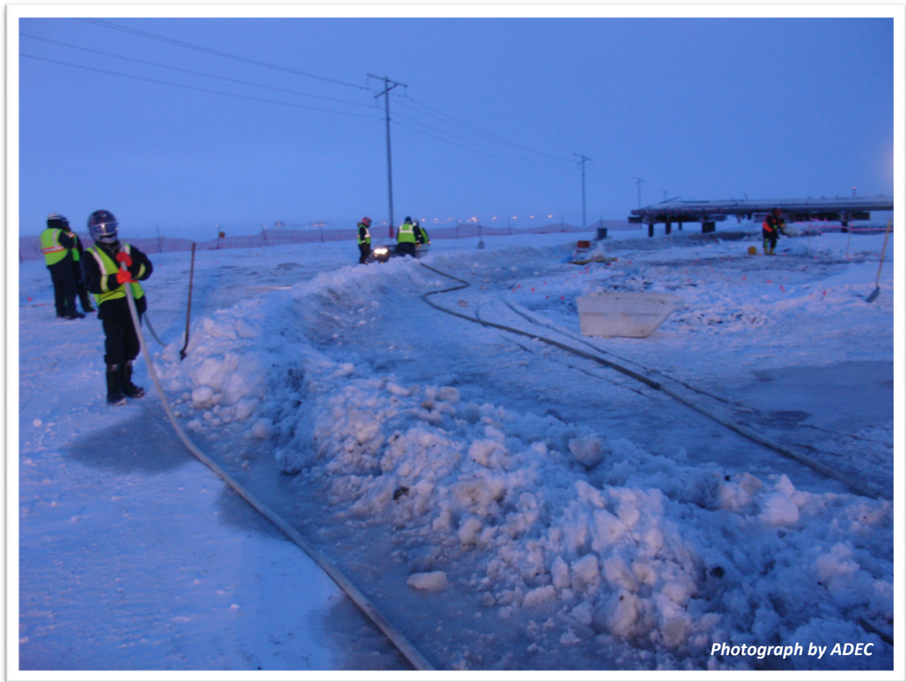
The day-shift crew building an ice berm around the spill site in preparation for steamer tactics.
