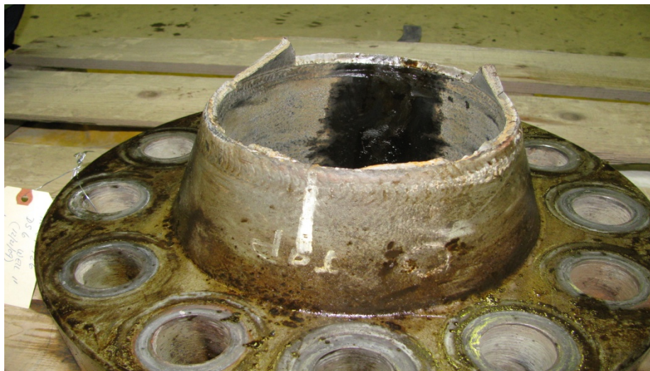
Break near flange
