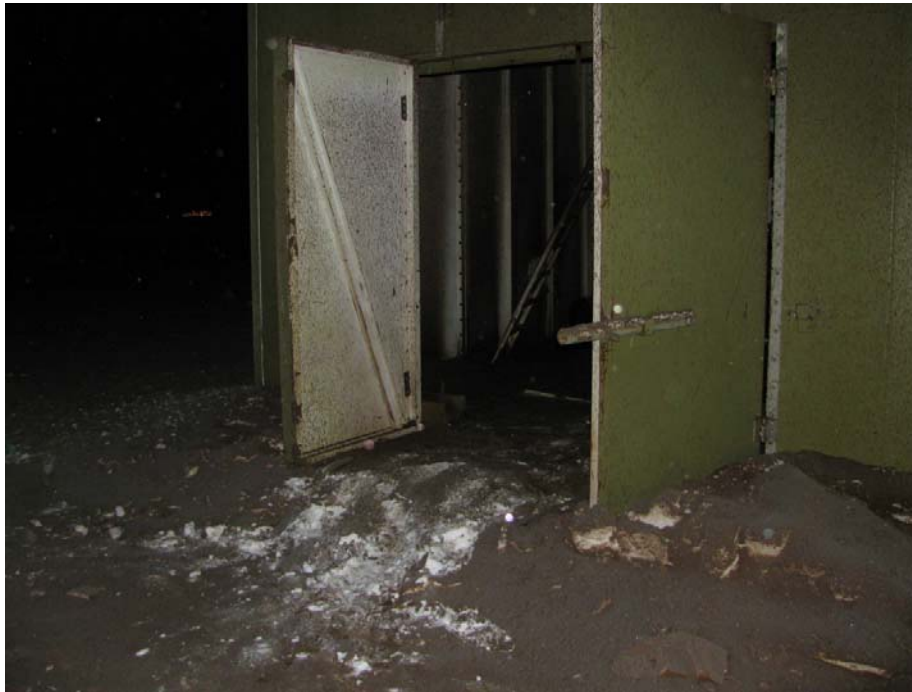
Contaminated and oiled snow outside of well house
