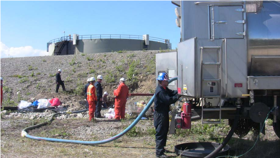
APSC crew pumping oil from the containment drainage pipe on May 27. (APSC photo)
