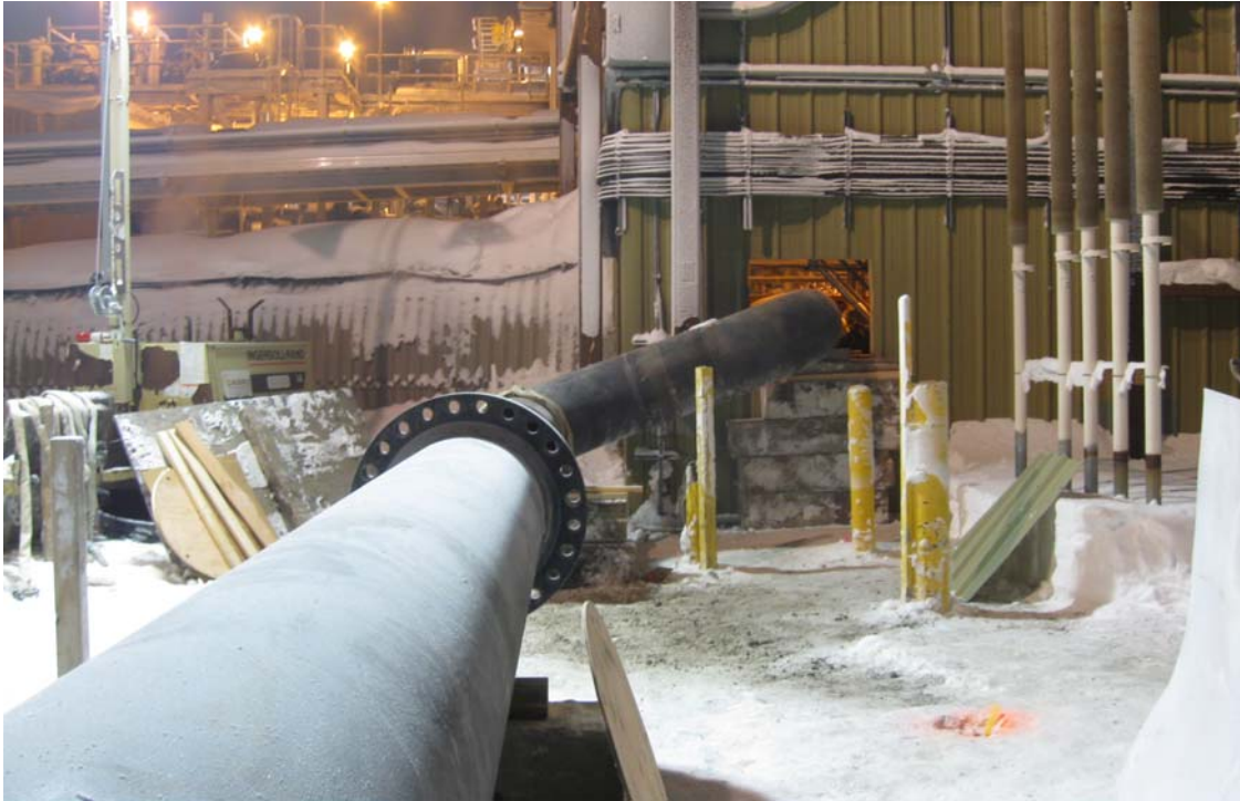
The 24-inch bypass line, under construction, enters the metering building ADEC photo 1/14/2011
