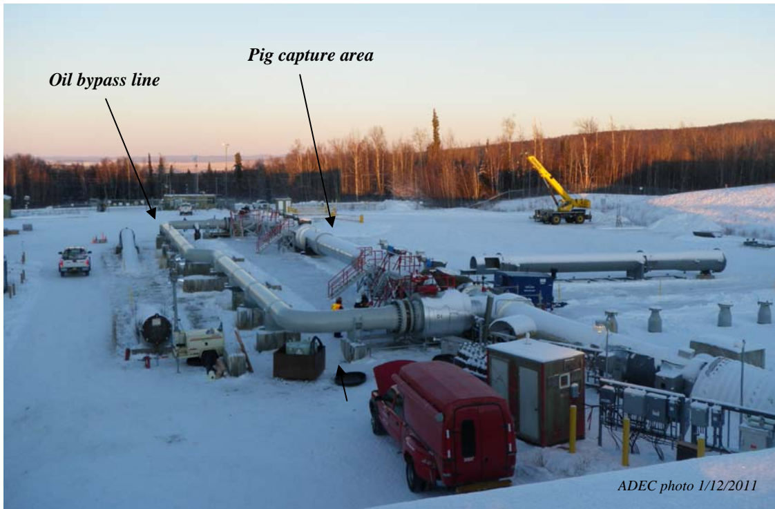
The section of pipe at Pump Station 8 in which the northern pig was trapped and the bypass line through which oil is being diverted around it ADEC photo 1/12/2011
