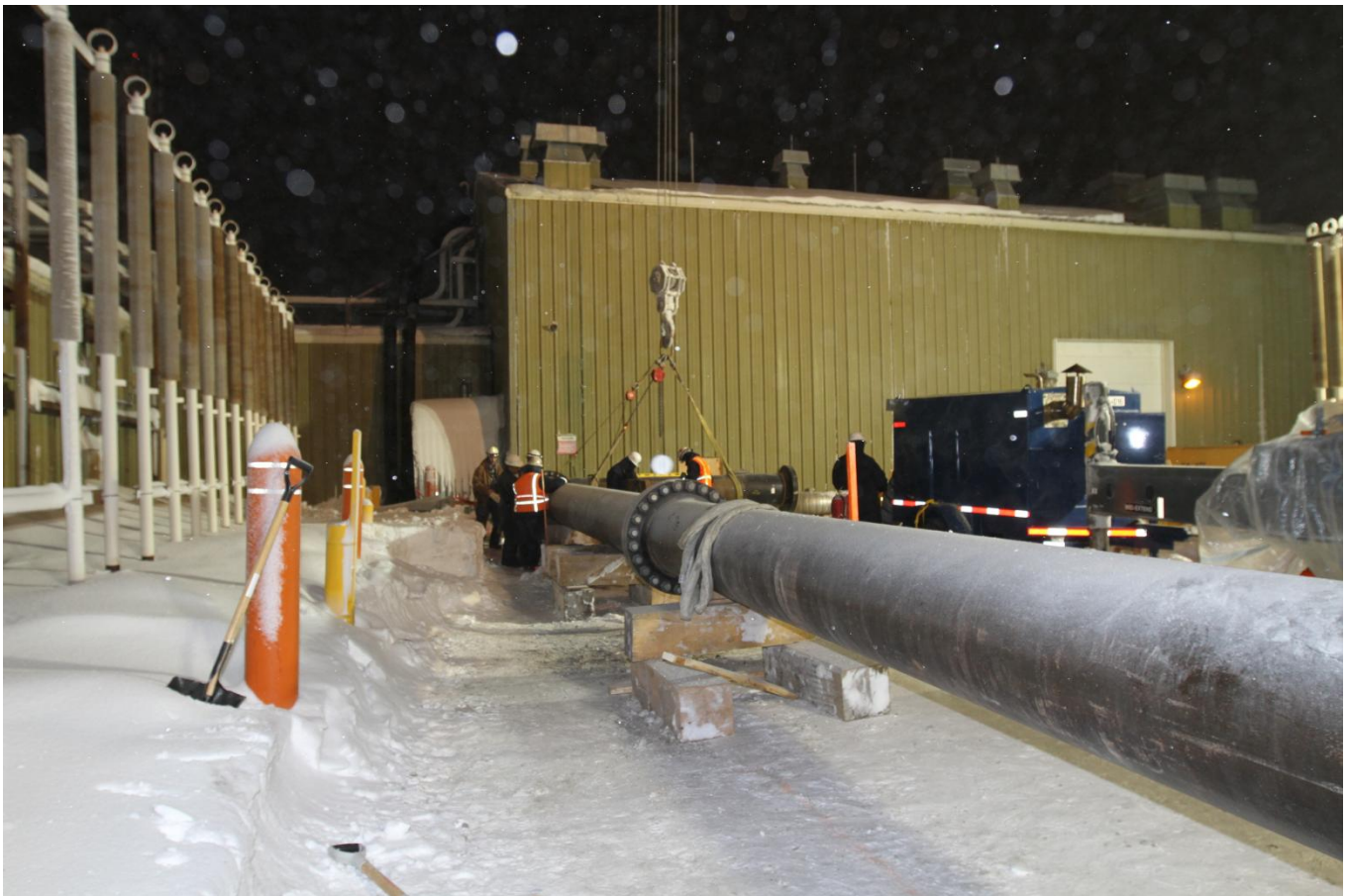
Workers at Pump Station 1 attach a section of pipe for the bypass pipeline. The 157-foot bypass pipeline was fabricated and shipped in sections from Fairbanks and assembled at Pump Station 1, about 500 miles north of Fairbanks.
