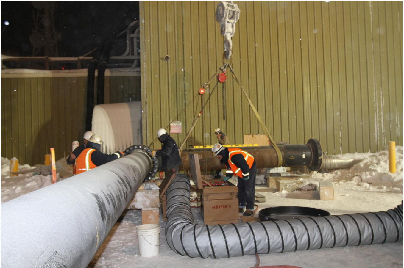
Workers at Pump Station 1 are fitting the next section of 24-inch diameter pipe to the recently assembled bypass line at Pump Station 1. This new line will bypass existing pipe, where a leak was discovered on January 8, 2011, and reroute crude oil around to the booster pump building.
