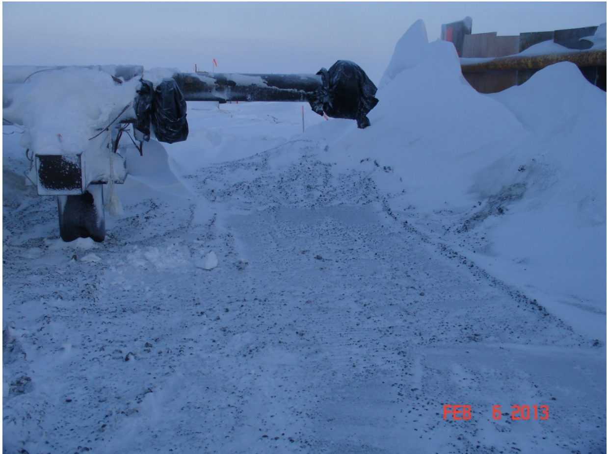
Lisburne Production Center L-1, eight inch test header pipeline – above ground crossing. (ADEC Photo)
