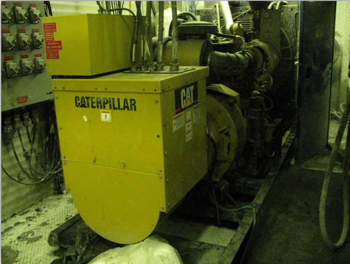
The cold start generator of the drill rig undergoing cleaning. ADEC Photo.
