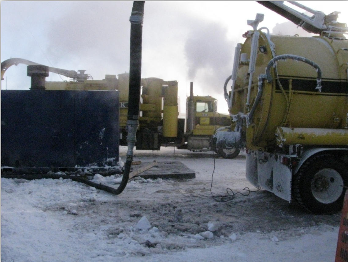
Supersuckers recovering mud and water from the steam thawing and cleaning operation. ADEC Photo.
