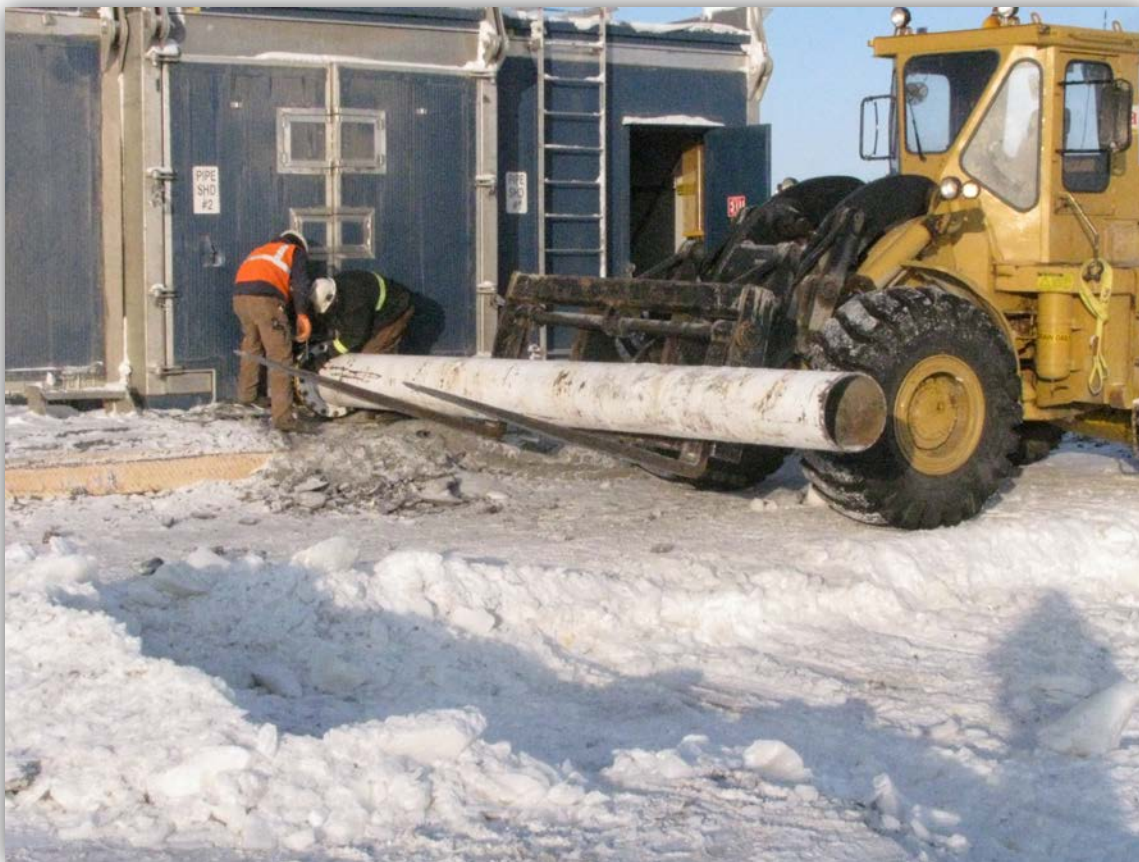
Crews installing piping on end of the gas diverter line. ADEC Photo.
