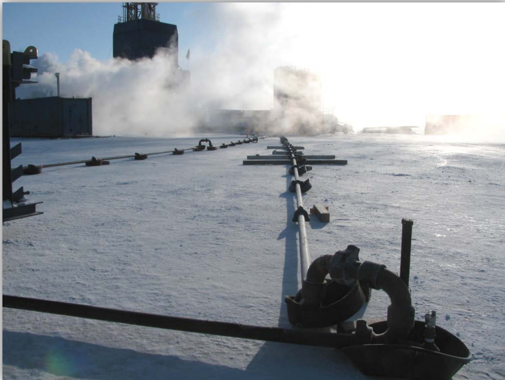
Piping used for moving mud and cement to the well for the well control operation. ADEC Photo.
