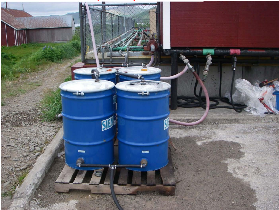
Filter system outside Peter Pan Seafoods secondary containment. Photo provided by Peter Pan Seafoods.
