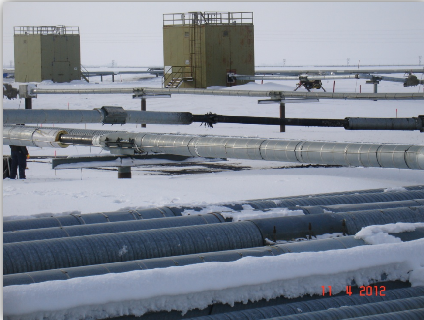
Drill Site 1 Well 11, eight-inch seawater injection pipeline failure. Viewing southwest over the reserve pit. (Photo/ADEC)
