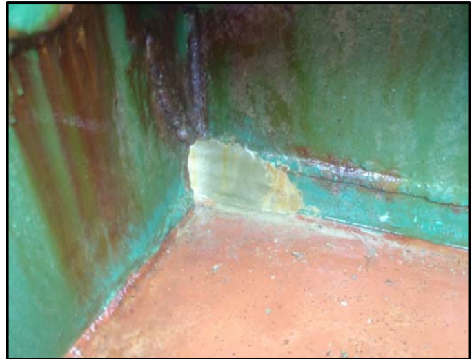
Temporary seal over the fractured area stopping the leak, September 13, 2012. (Photo/ADEC)
