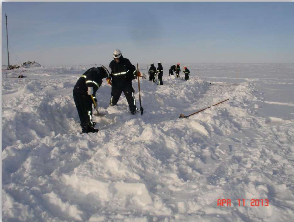
Spill cleanup technicians removing contaminated snow from the snow-covered tundra, April 11, 2013. (Photo/ADEC)
