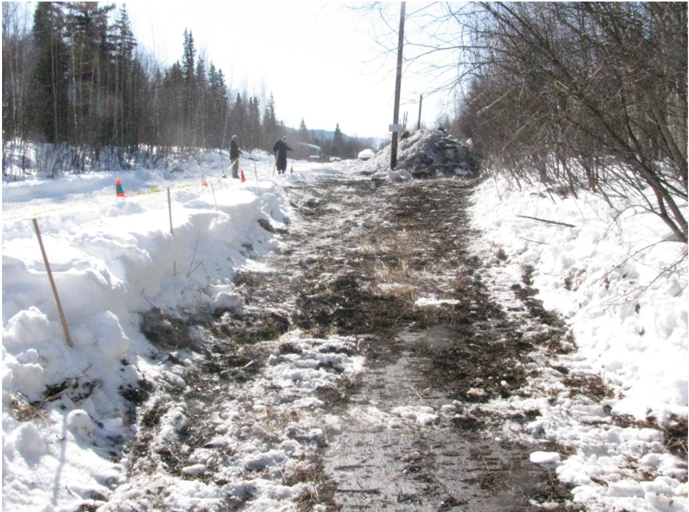
Spill site showing contaminated snow stockpiled for placement into portable tanks, April 17, 2012. (Photo/ADEC)
