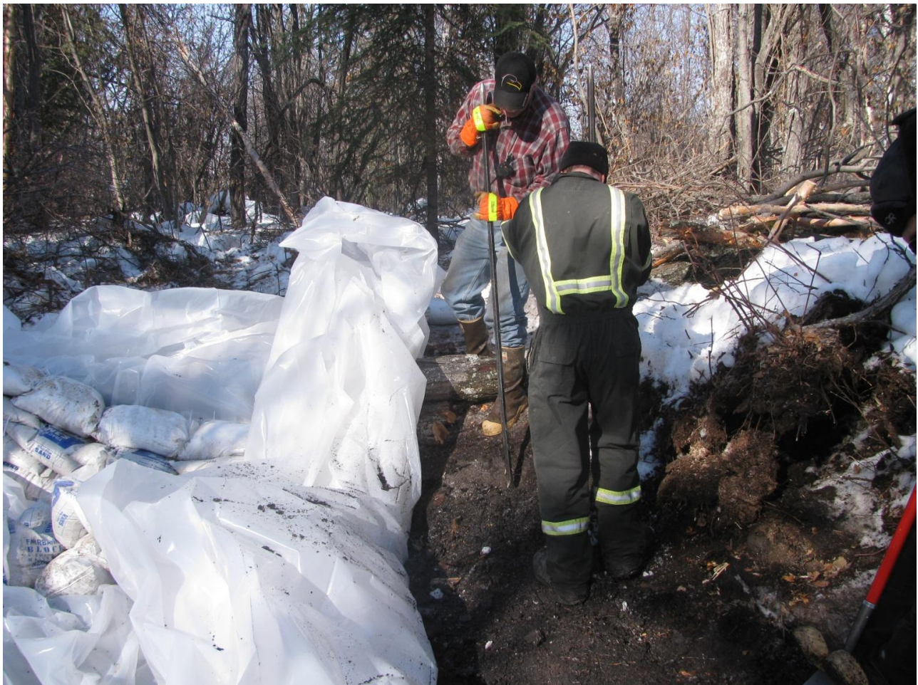
ADEC Photo of spill site showing an Emerald and a local responder constructing the underflow dam used to manage runoff and melt water from the site.
