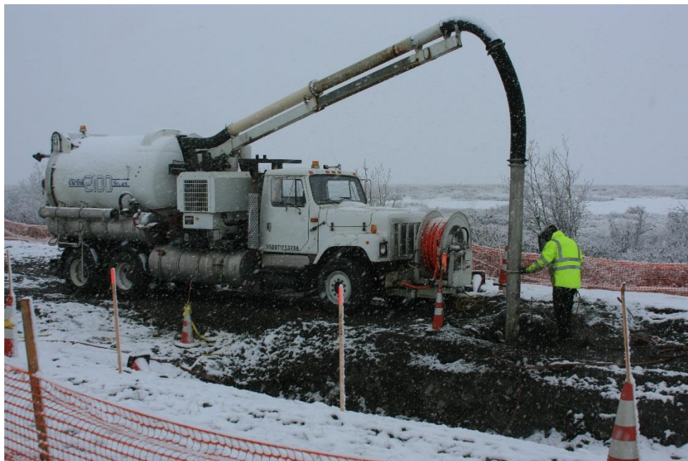
Cleanup crew using a vacuum truck to uncover TAPS utility lines, May 13, 2014. (Photo/ADEC)
