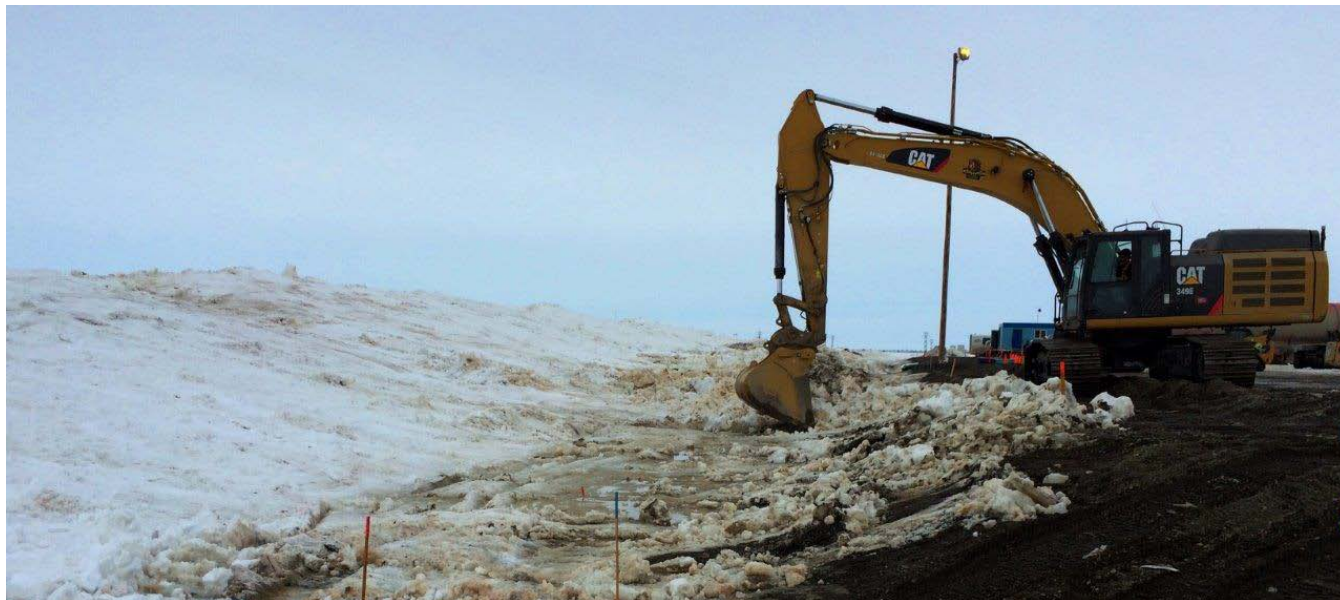
An excavator with a smooth-lip bucket removes contaminated snow from an off-pad snow berm, May 1, 2014. (Photo: ADEC) This operation was noted in sitrep #3
