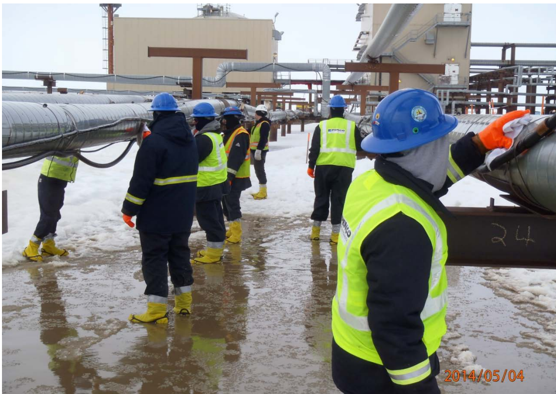
Cleanup personnel remove oil sprayed onto well piping during the April 28 H Pad Well 8 flowline rupture. May 3, 2014 (photo: Fritz, ADEC)
