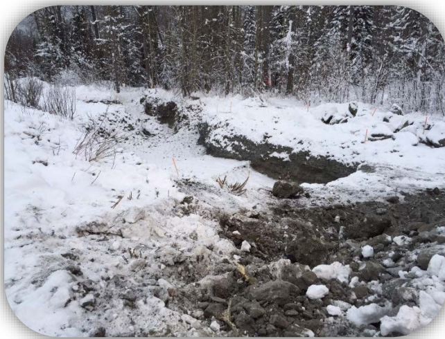
Excavation of contaminated gravels at the end of Phase 1 Operations Photo take 12/22/2014 by ADEC
