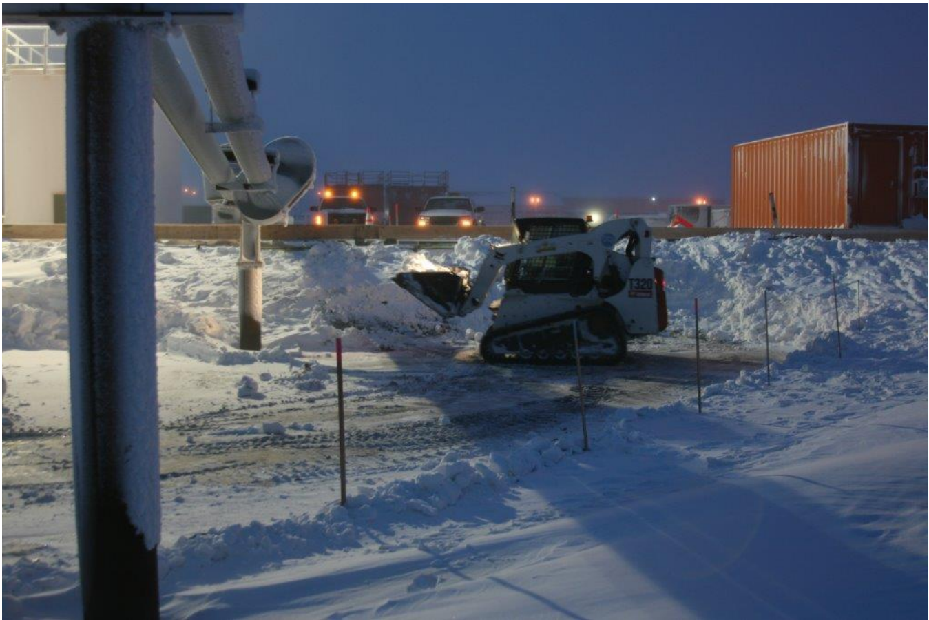
ACS removing contaminated snow from the reserve pit, December 16, 2014. (Photo by Paul Lhotka/ADEC)
