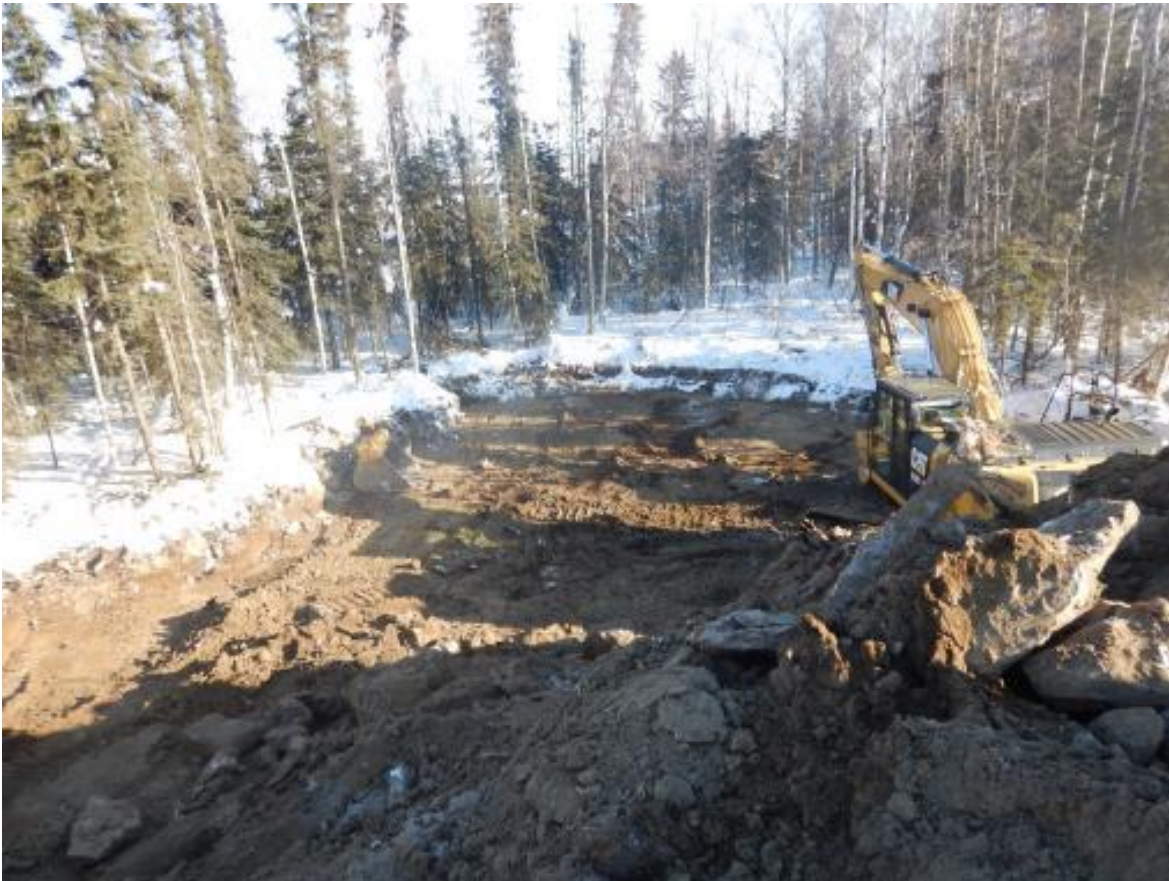
Picture of delineated spill area, facing northeast, during the removal of affected resources (Photo/ERM Alaska, Inc.)
