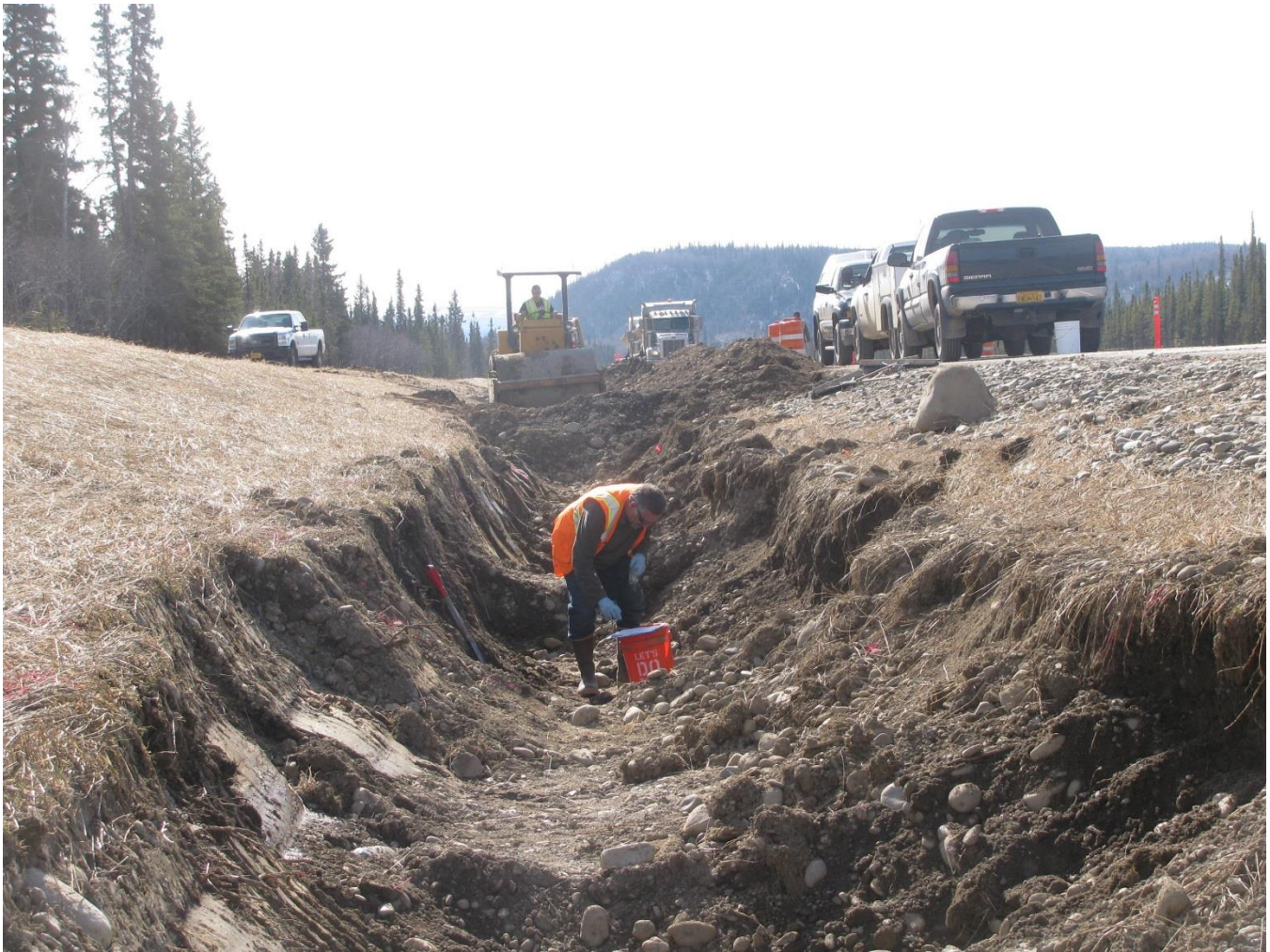
Figure 1. Environmental contractor field screening material from the ditch on the east side of the Parks Highway on April 25, 2015. (Photo/ADEC-Ghormley)
