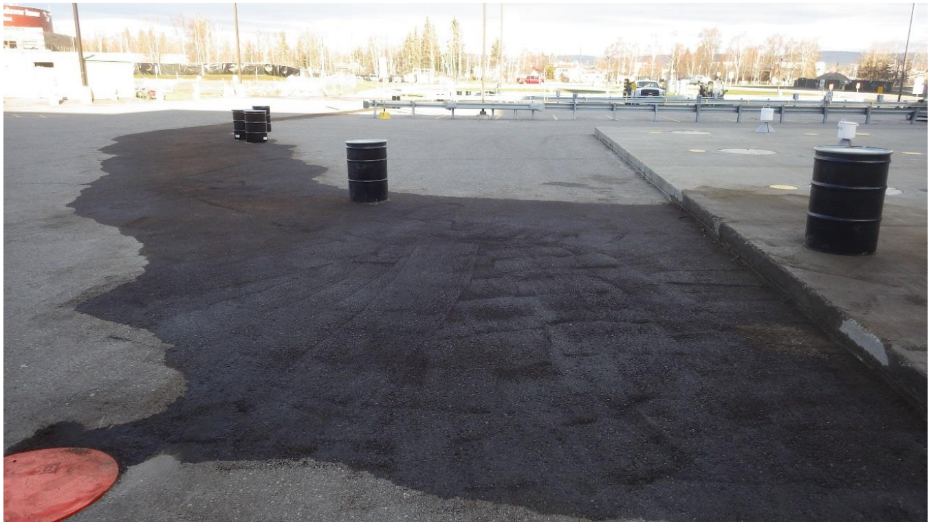
Figure 2. Drummed contaminated absorbent material along the swept spill path in the FMH parking lot. Secured sewer manhole cover can be seen in the bottom left-hand corner. Photo: Patrik Sartz/ADEC.
