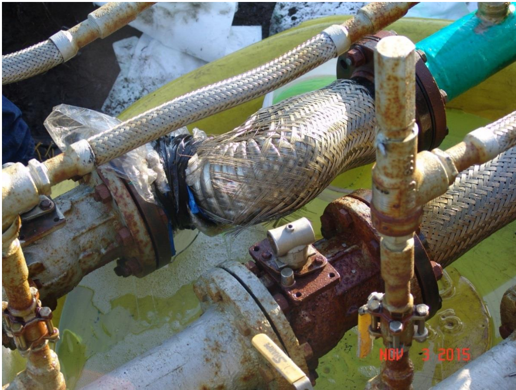
Nov. 3, 2015, Displaced and ruptured flexible pool coupling. Photos by Frosty Fuels, LLC.
