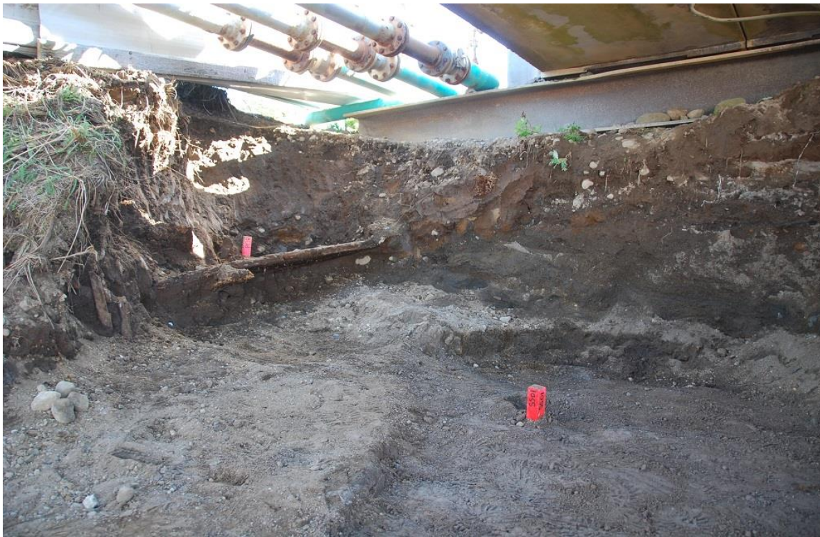
Close up of excavation under Cold Bay Dock, June 21, 2016. (Photo/ Kanaga Environmental Consulting LLC)
