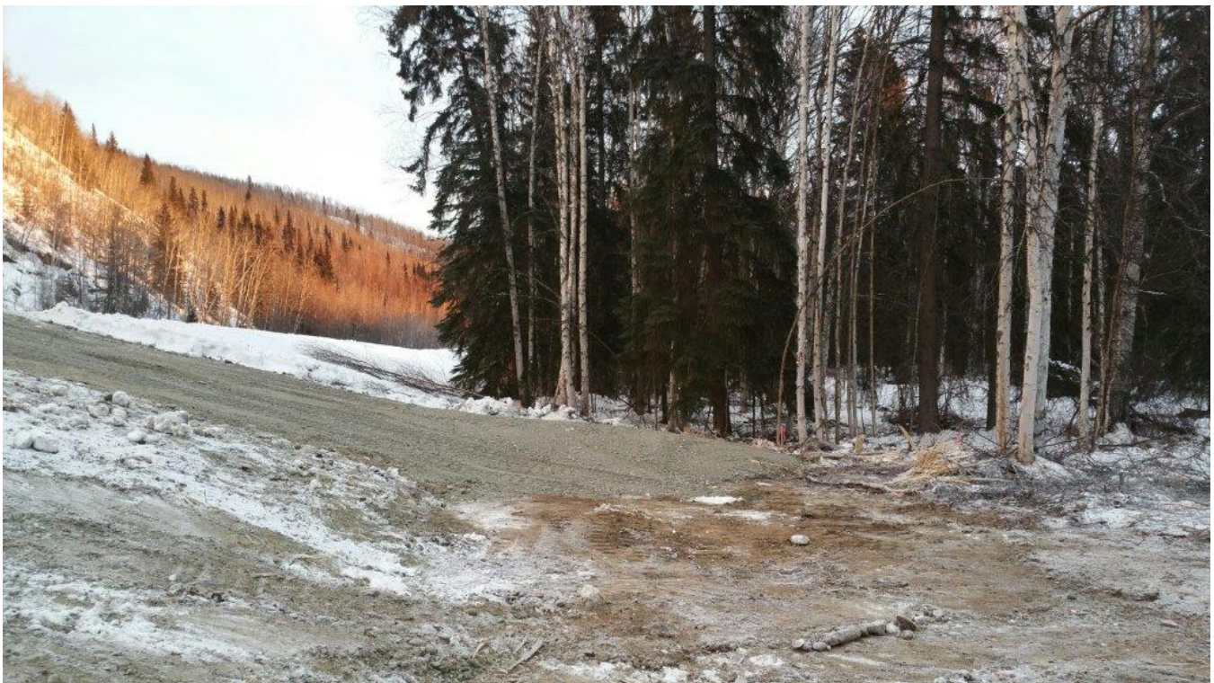
Figure 1. Spill area with a "cap" of clean fill two feet deep. [Photo: RSE]
