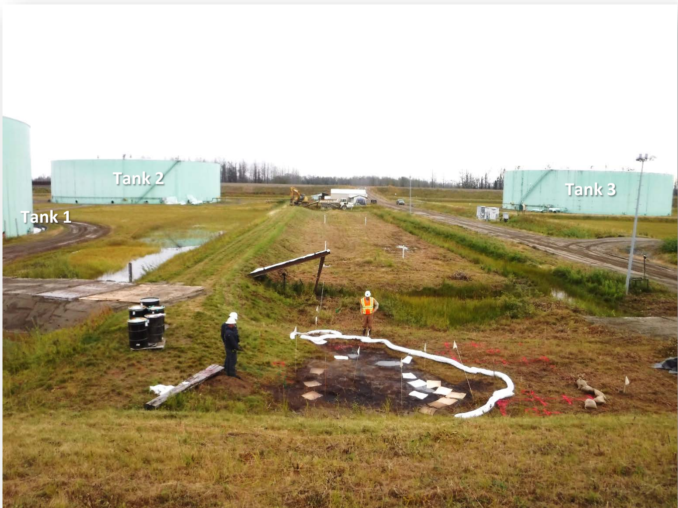
Photo 1: Foreground - Surface stain above buried flanges between tanks 1 and 4, which was discovered and reported on July 28, 2016. Background – Delineation activity where free product was observed, August 10,
