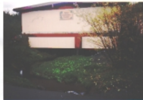
Figure 12: Wrinklneck Creek channel under structure on Monastery Street (City and Borough of Sitka photo)
